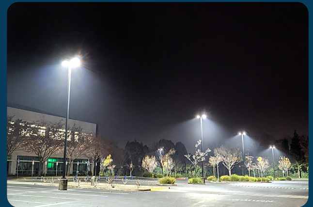
Altech's LED Hyper Series Area Lights were the perfect lighting solution for maximizing savings and providing a uniform distribution of light for Sunnyvale Business Park.
